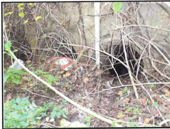
Existing Pipe Blockage on Western End
