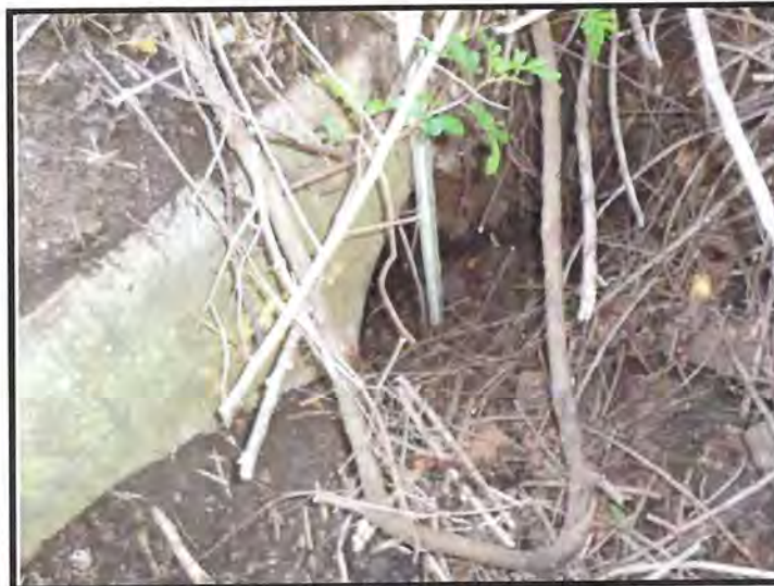
Existing Partially Blocked RCP and Endwall on Eastern End
