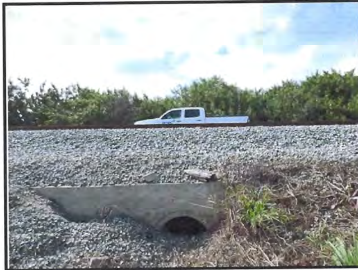
Eastern Headwall at MP 177.03A. Double 36" RCP with One Completely Blocked and One 60% Blocked.
