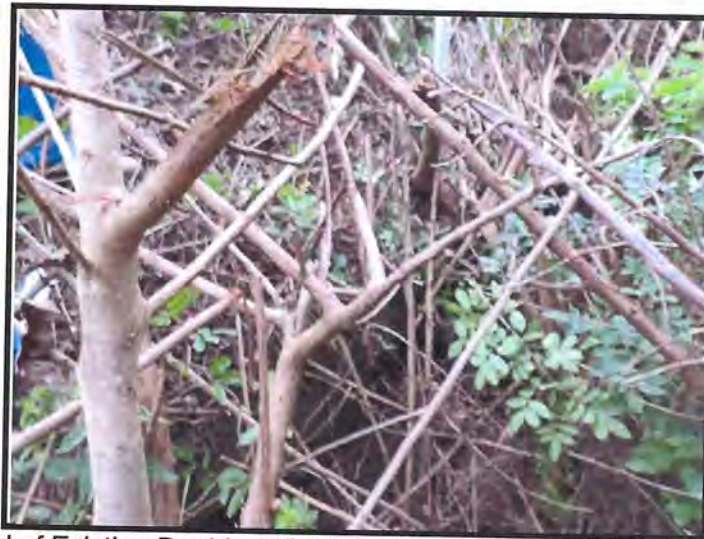
Western End of Existing Double 30" RCP. Note: Severely Overgrown Vegetation
