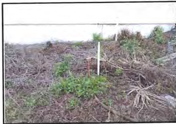
Survey Rod and Probe Mark the Approximate Western End of Existing Double 18" RCP. Note: Also the Lack of Any Defined Trackside Ditch and the Proximity of the Adjacent Building.
