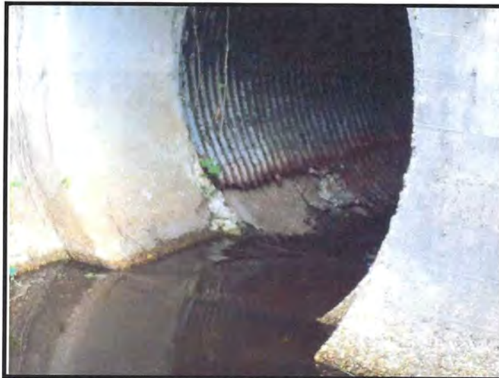
Looking at Southernmost Culvert at the West End Showing Corroded CMP Inside RCP.
