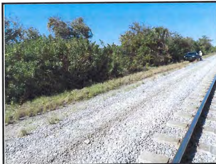
MP 193.32 Overgrown West (Upstream) Ditch
