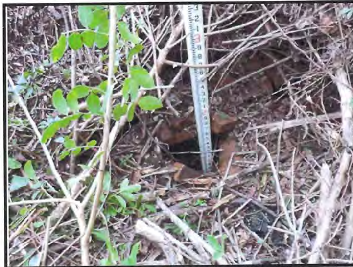
Existing Broken Terra Cotta Pipe and Blockage on Western End
