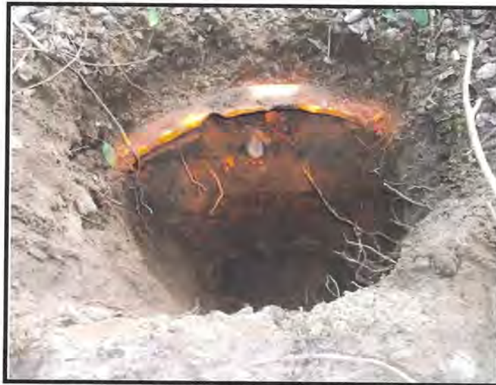
Existing Western End of Buried Culvert at MP 173.90 Note: It is 100% Blocked
