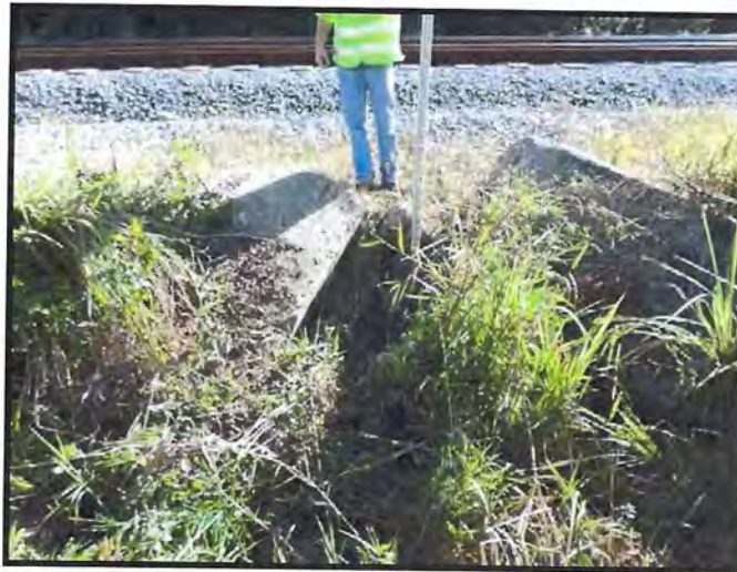
Severely Damaged/Non-functioning Endwall and Damaged West End of Cross Drain MP 210.97
