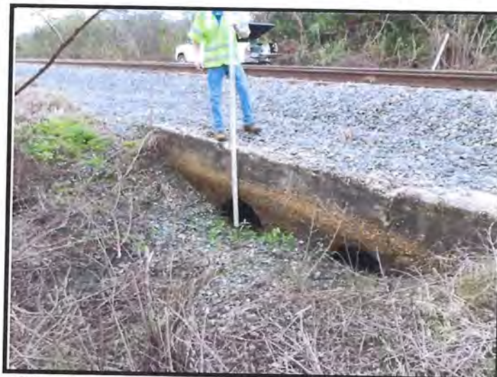
Eastern End of Existing Endwall and Double 30" RCP Estimated at 60% Blockage
