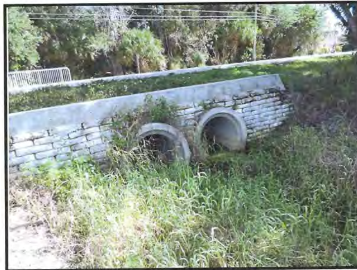
Receiving (East) Ditch and Double 42" Cross Drains Under CR 5A
