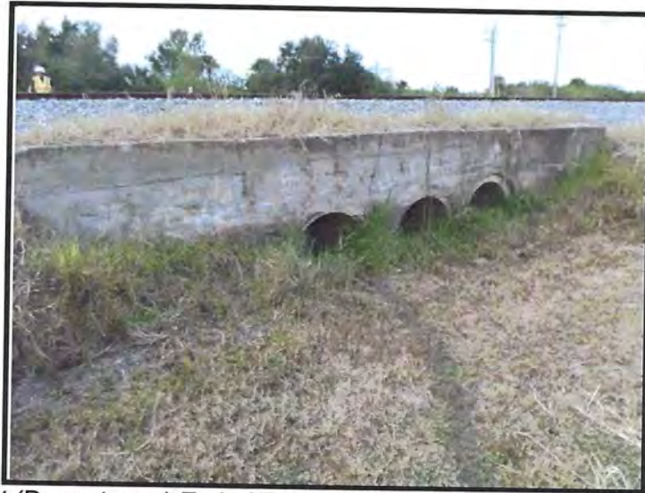
East (Downstream) End of Triple 30" RCP Culverts at MP 226.26. Note: The Severely Cracked Endwall.
