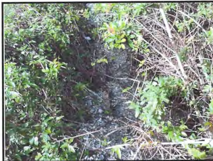
East (Downstream) End of Double Culverts at MP 205.90. Note: The Severe Blockage of Both Culverts.
