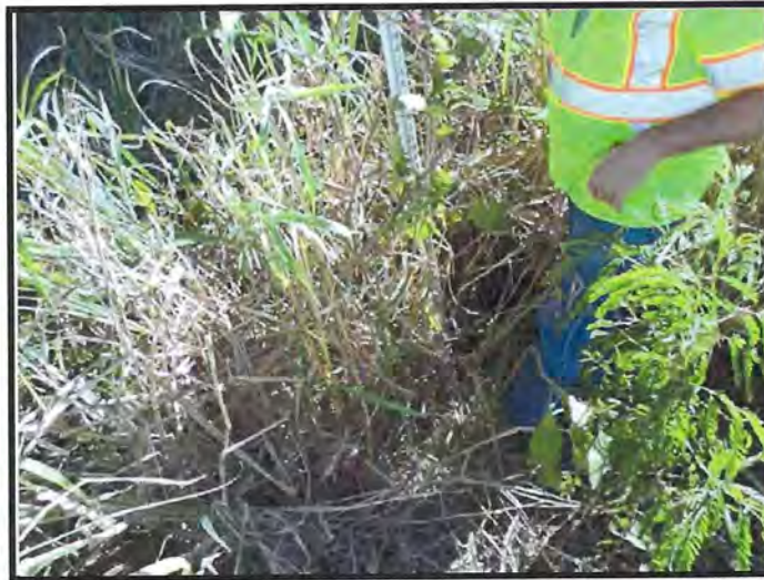
East (Downstream) End of Double 30" RCP Culverts at MP 204.30. Note: The Severely Overgrown Vegetation.
