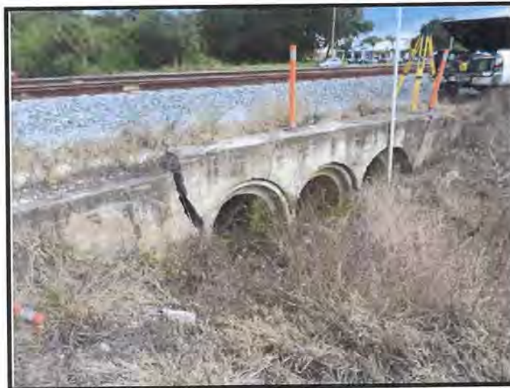
West (Upstream) End of Triple 30" RCP Culverts at MP 226.26. Note: The Severely Cracked Endwall.
