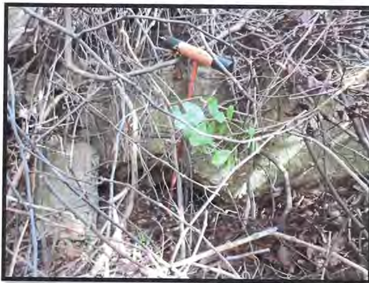
Existing Pipe Blockage on Western End (Current Culvert is Non-functional)
