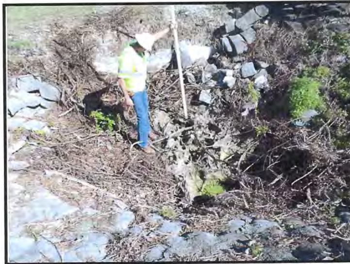
Looking Toward Track at Existing Sump Upstream (West) End of MP 214.85 Cross Drain. Note: The Survey Rod is at the end of the Collapsed CMP Extending from Headwall into Sump.
