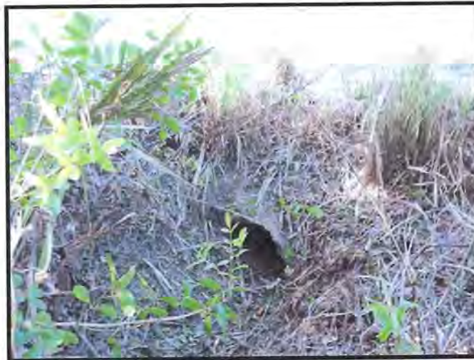
East End of Cross Drain MP 210.97 and Sediment Accumulation
