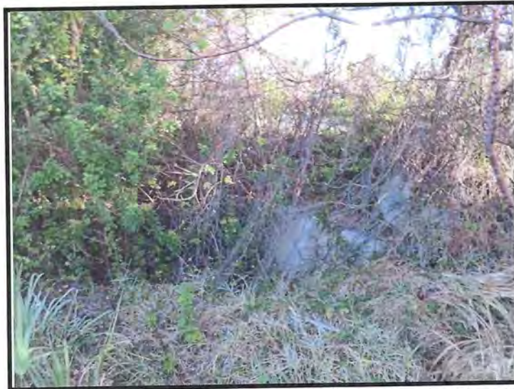
West End of Cross Drain MP 208.87. Note: Excessive Vegetation
