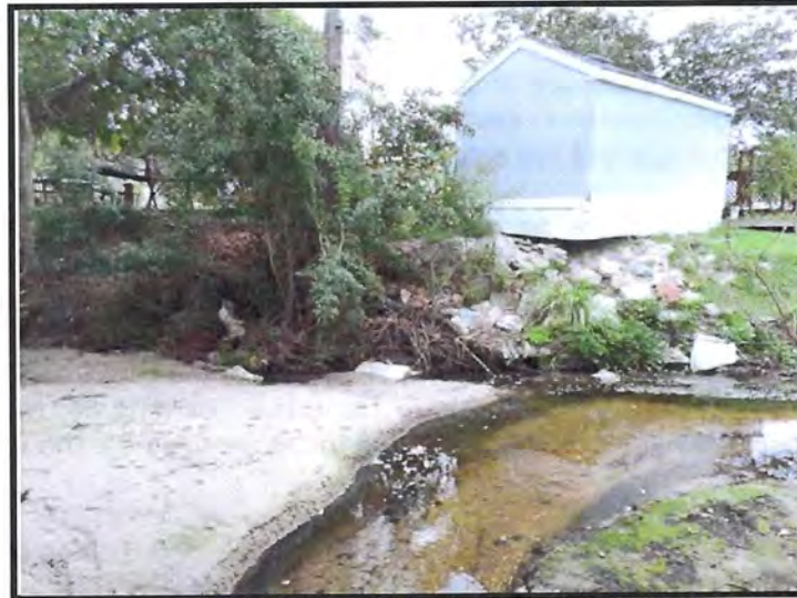
Existing Erosion at Existing Structure East (Downstream) of Culverts and Weir
