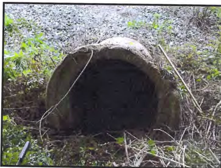
Existing Damaged West End of Cross Drain at MP 231.27
