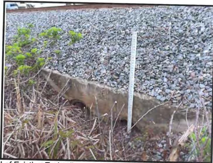
Eastern End of Existing Endwall and Double 18" RCP Estimated at 80% Blockage
