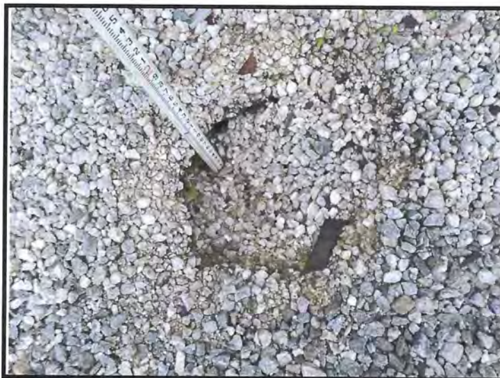
Void Over Middle Culvert at MP 184.02 (Probable Joint Failure)
