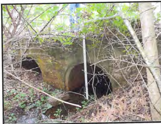
Eastern End of Existing Endwall and Double 48" by 53" Oval RCP. Note: Estimated 50% Blockage of Southern Barrel
