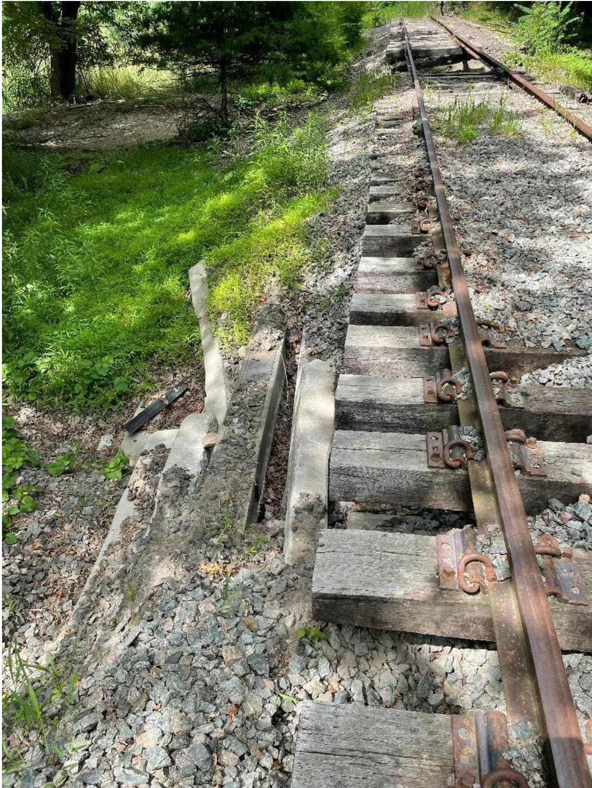
MP 6.71 Culvert, obvious shoring attempt, mouth plugged, stone dumped
