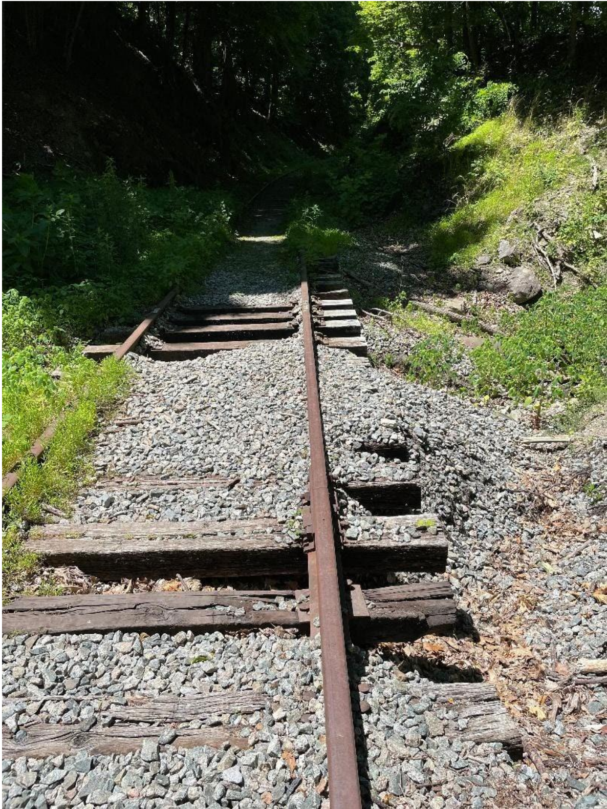
MP 3.82 culvert wash (left side of picture mouth plugged)
