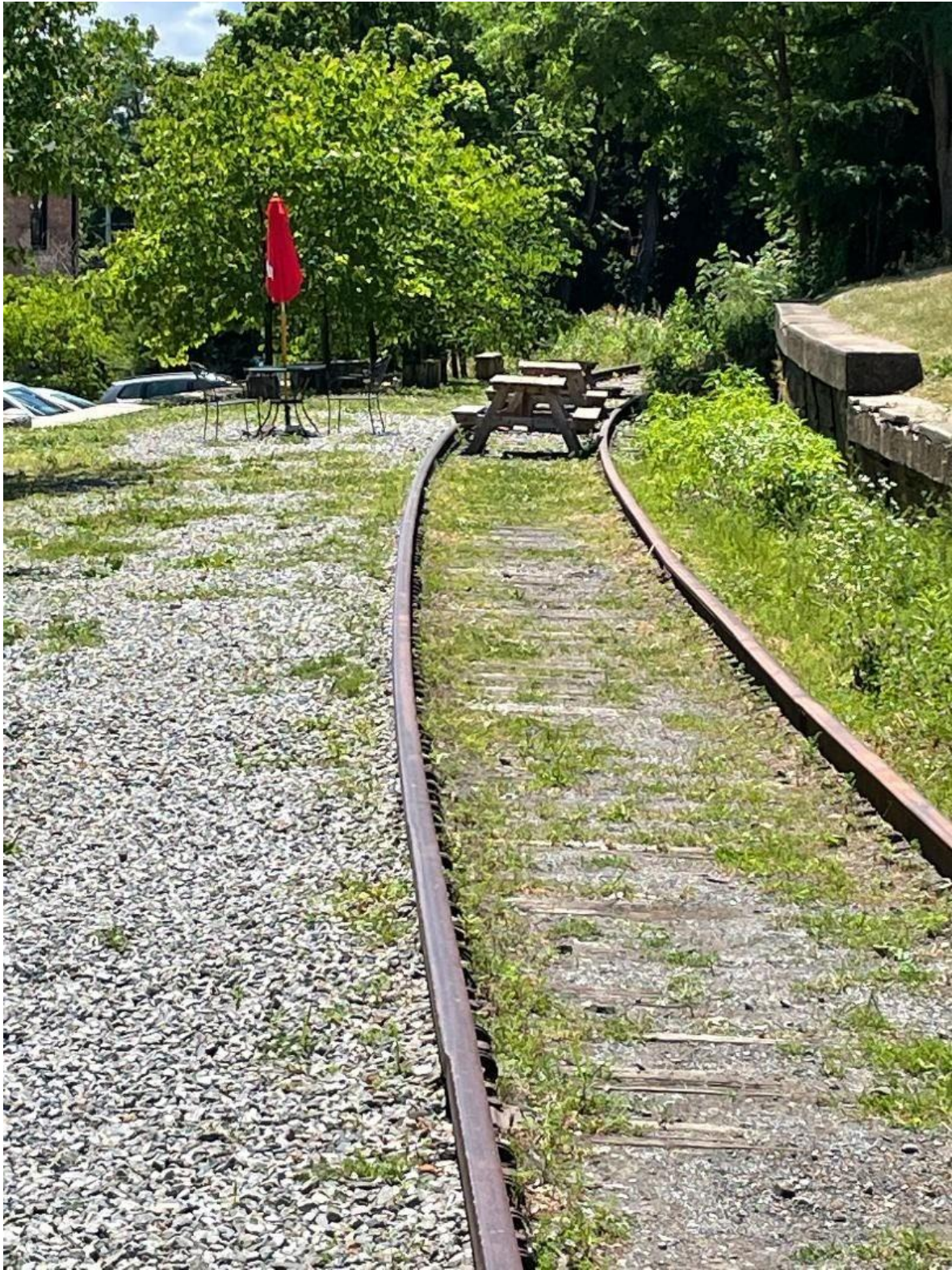
MP 2.17 East Main Street encroachment
