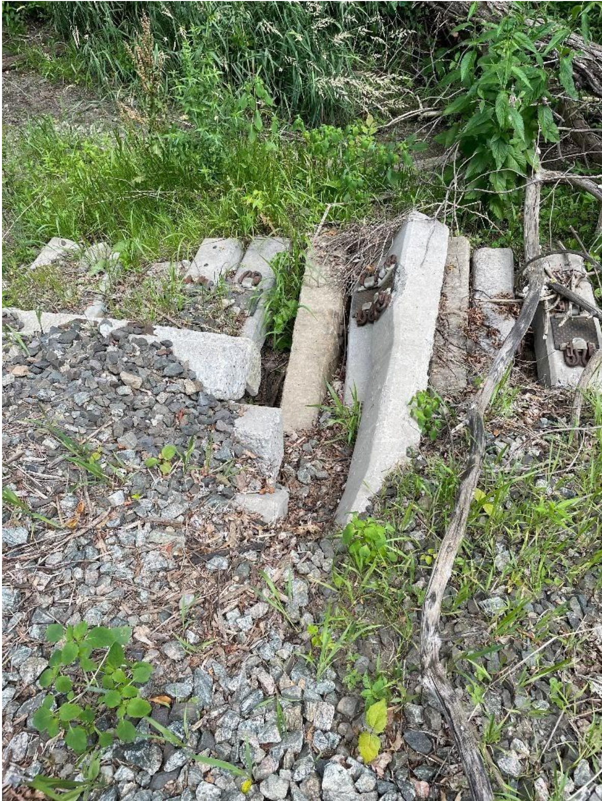
MP 6.62 Culvert mouth side, shoring looked older and in ditch, possibly leading to wash
