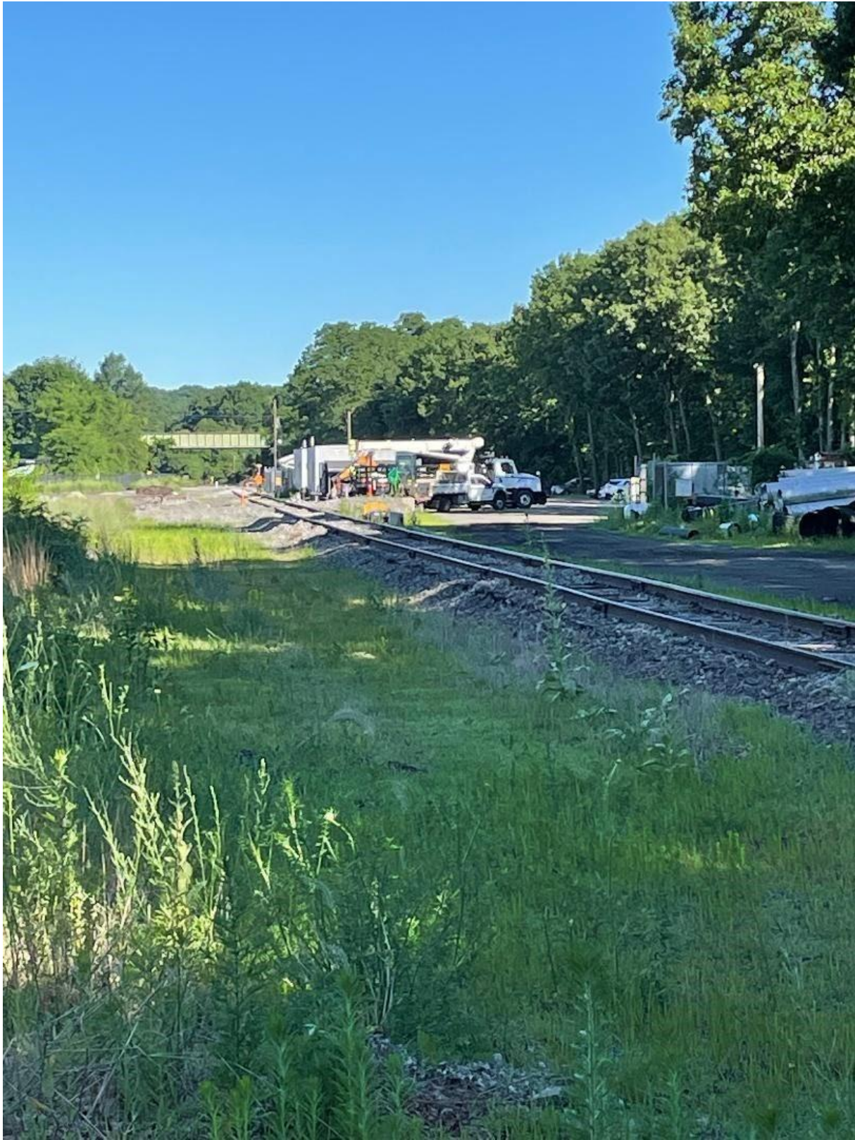
Hopewell Yard, Maintenance of Way facility, Track is disturbed significantly.
