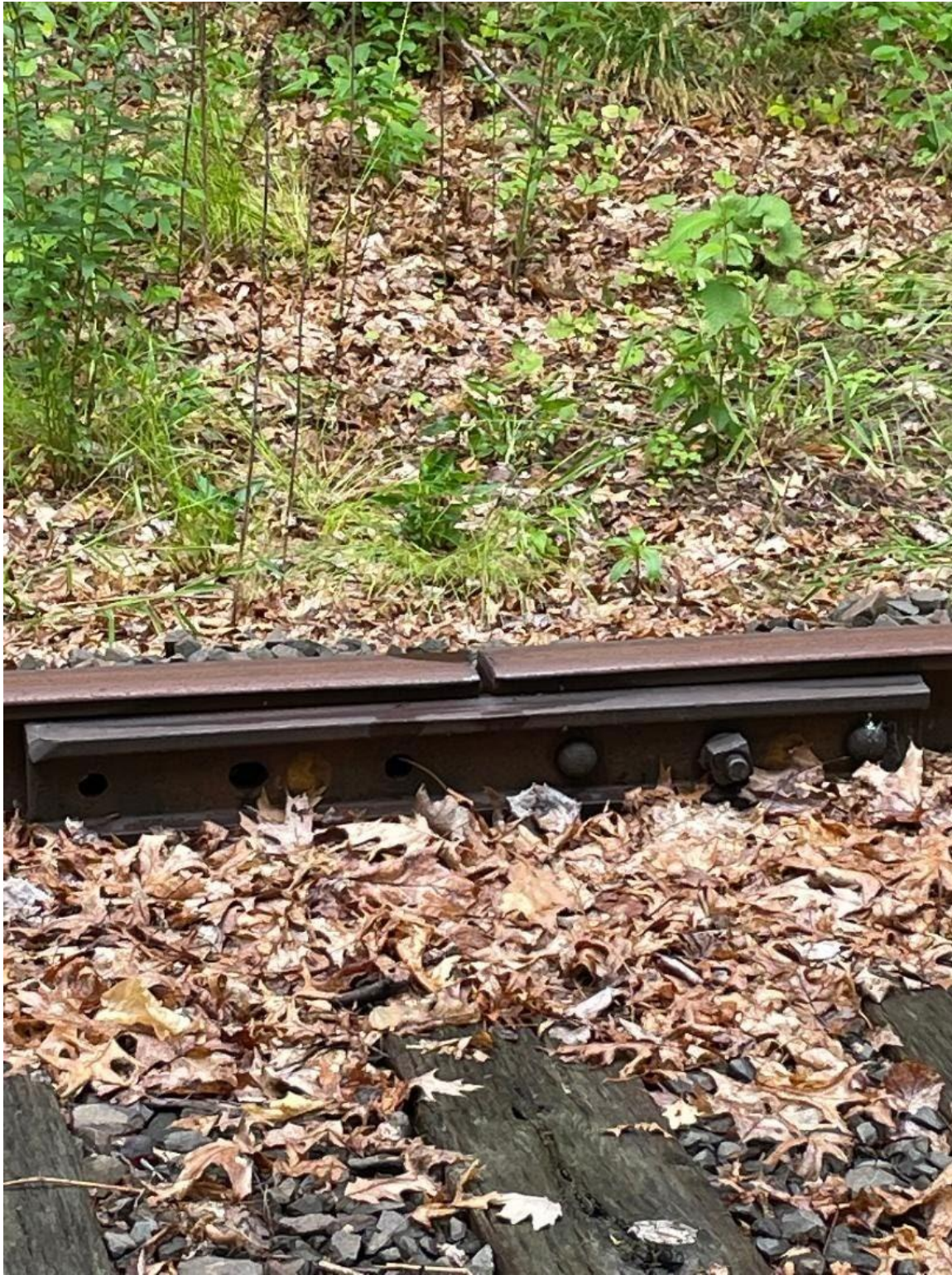
Example of bolt defects, areas found like this in different miles (couldn't find old missing bolts, areas were in groups and all on one rail end)
