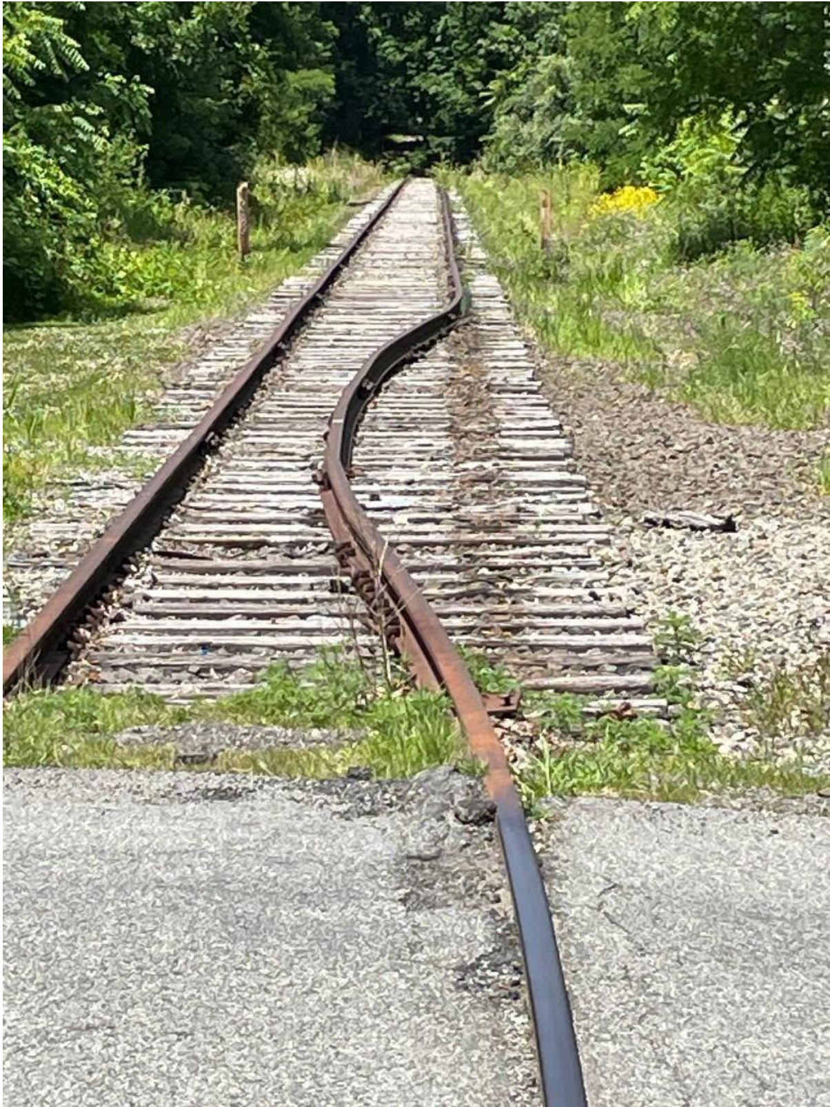
MP 4.10 just west of Washington Ave, rail not seated and plates missing.
