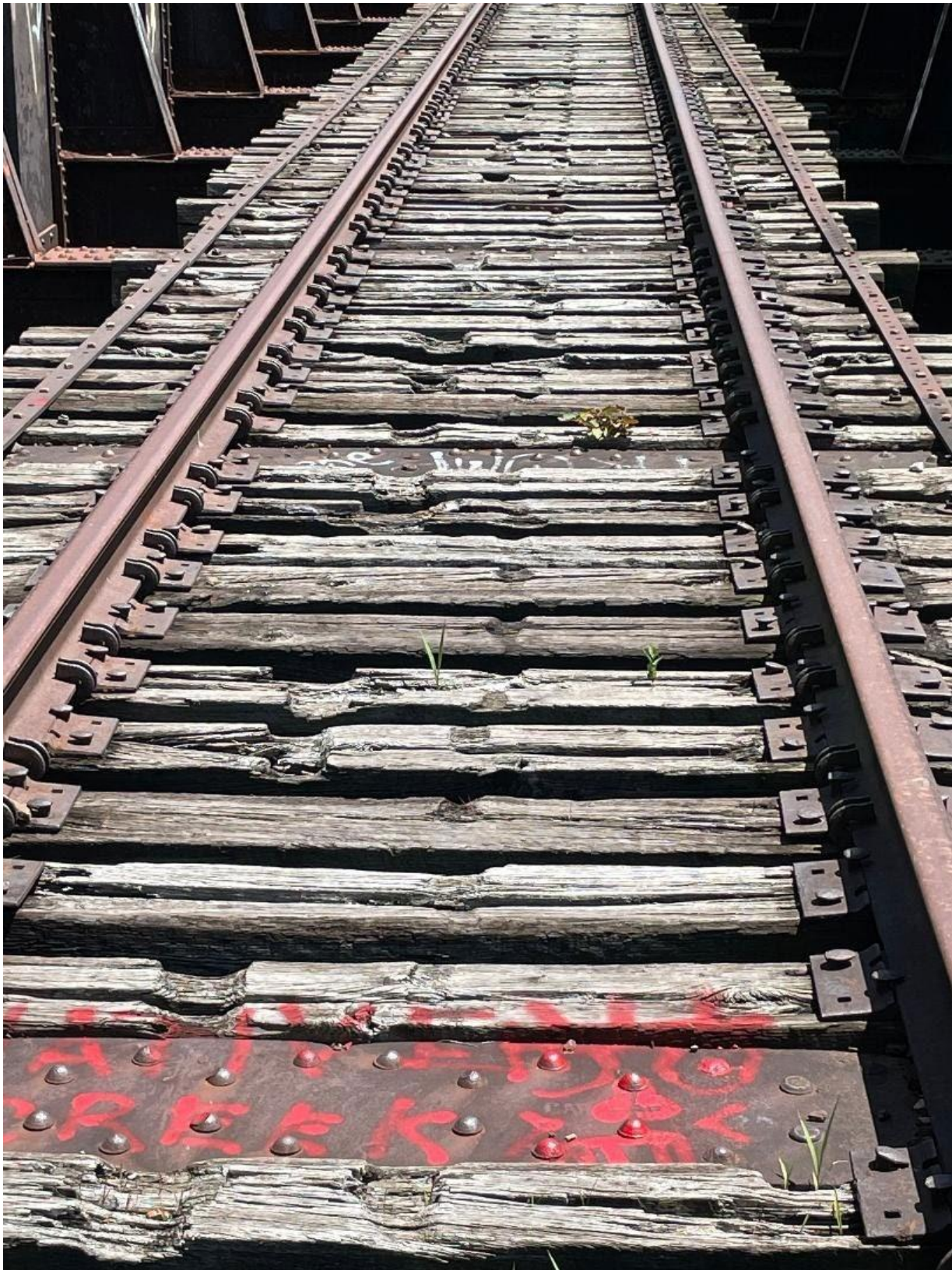
MP 0.63 Bridge Hudson Line, needs completely all new timbers
