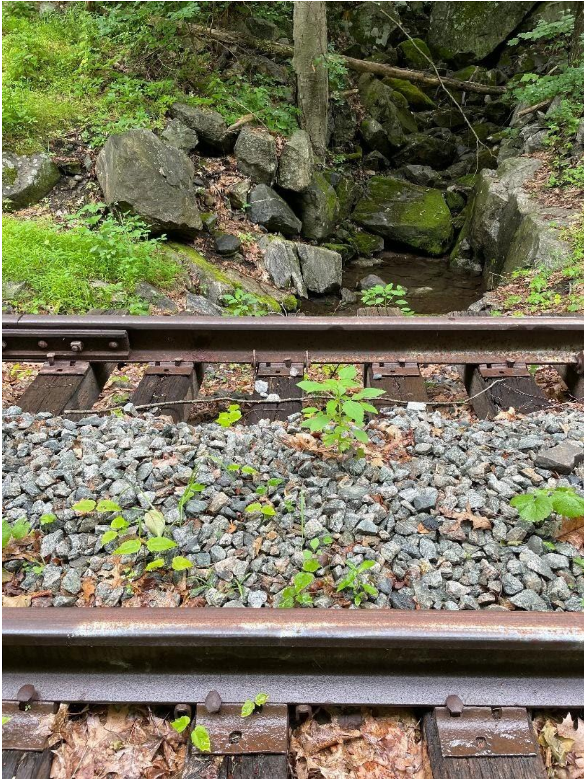
Small wash at culvert MP22.43, mouth is effectively blocked, stone in gauge.
