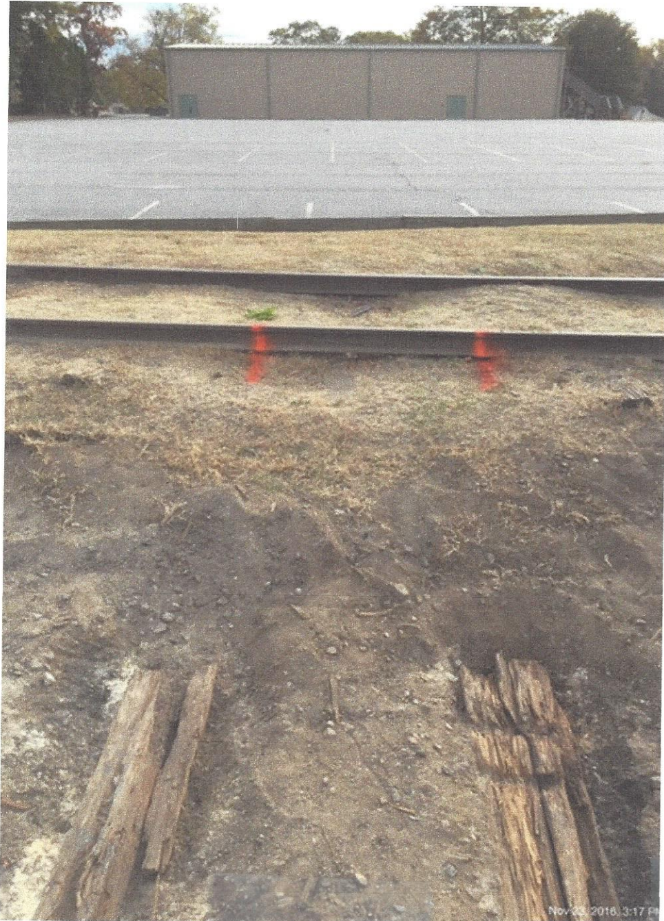
Photograph 26: Photograph of uncovered crossties and ballast located on Runaround Track right-of-way with GWRC Mainline Track in background, dated November 23, 2016
