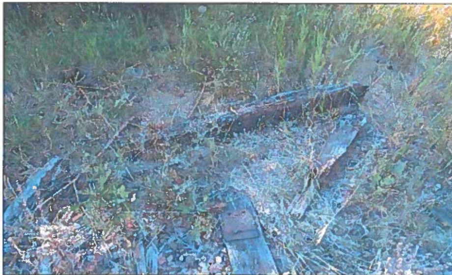
Figure 11. Broken railings and ties near south end, plan view.
