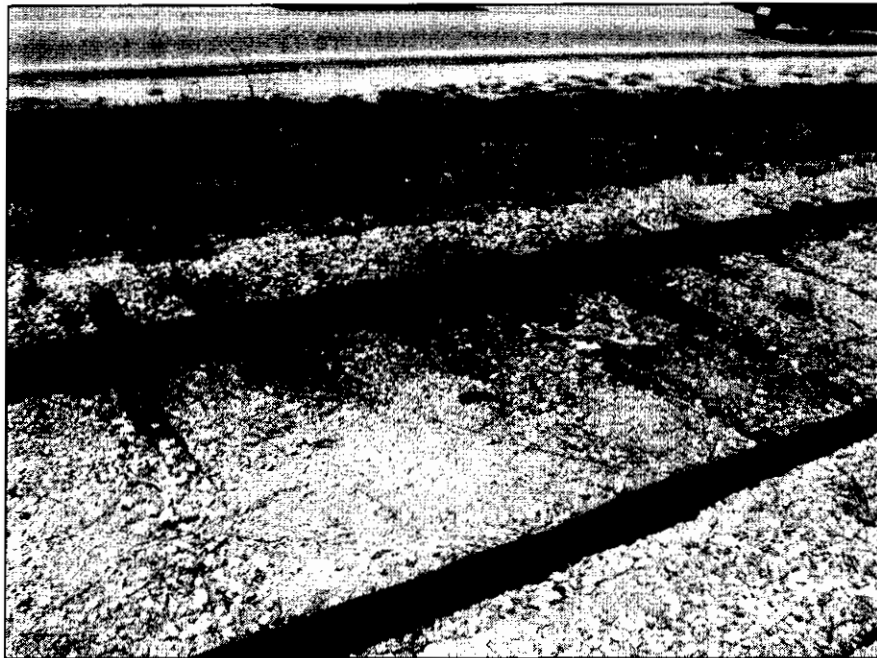
Typical Joint Area Exhibiting Poor Tie Conditions
