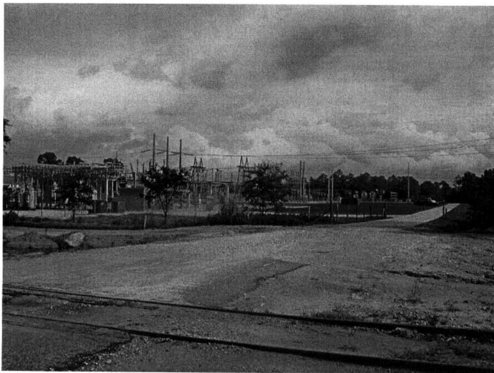
(4) FLORIDA POWER & LIGHT FACILITY LOOKING NORTH
