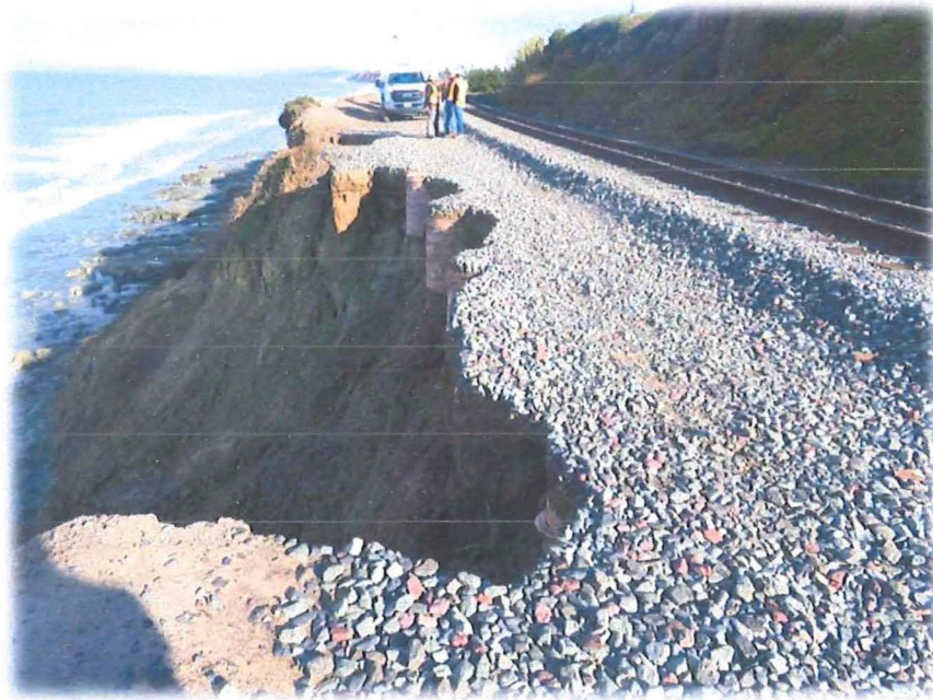
MP 244.25: Bluff Erosion west of Seagrove Park looking North
