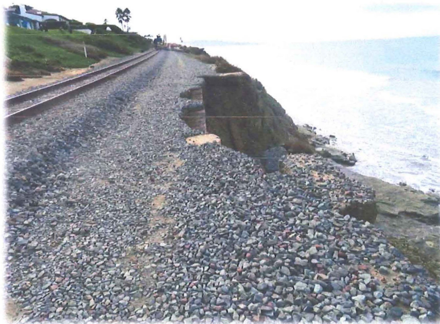
MP 244.25: Bluff Erosion west of Seagrove Park looking South
