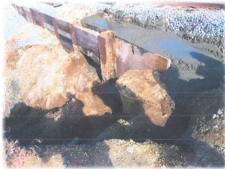
MP 244.30: Wash Out Erosion Repair SW of Seagrove Park
