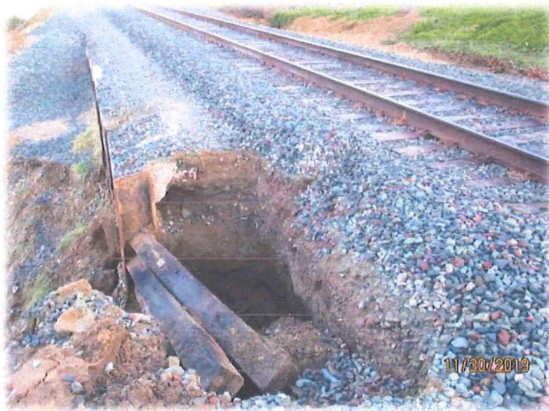
MP 244.30: Wash Out Erosion SW of Seagrove Park
