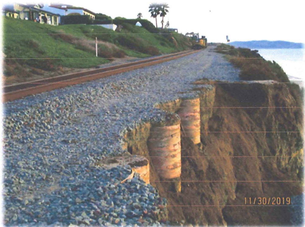
MP 244.25: Bluff Erosion west of Seagrove Park
