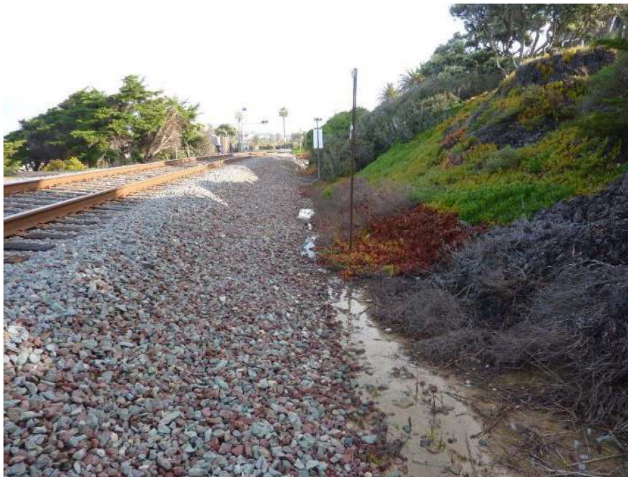
Drainage ponding along side of track
