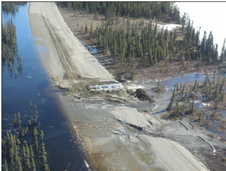
Figure 2: Aerial photograph at STA4605 looking at the grade washout on project right toward Muleshoe Lake (the bright white, upper-right corner of the photo). April 21, 2014.
