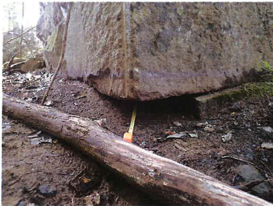
Photo 8: Undermining of center pier
