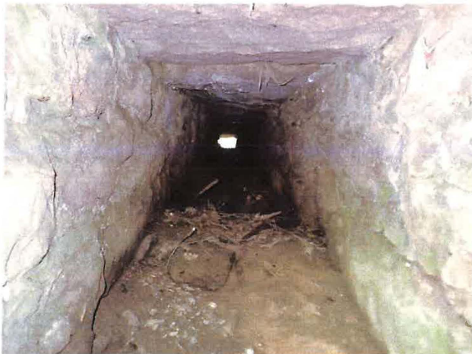
Photo 48: Interior of Culvert 10 with Void in Ceiling
