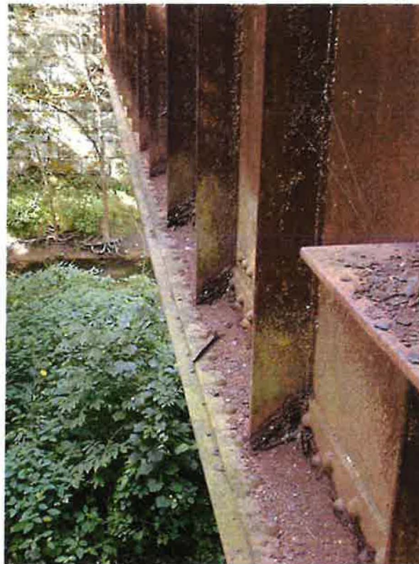
Photo 10: Rusting and deterioration of the steel stiffeners
