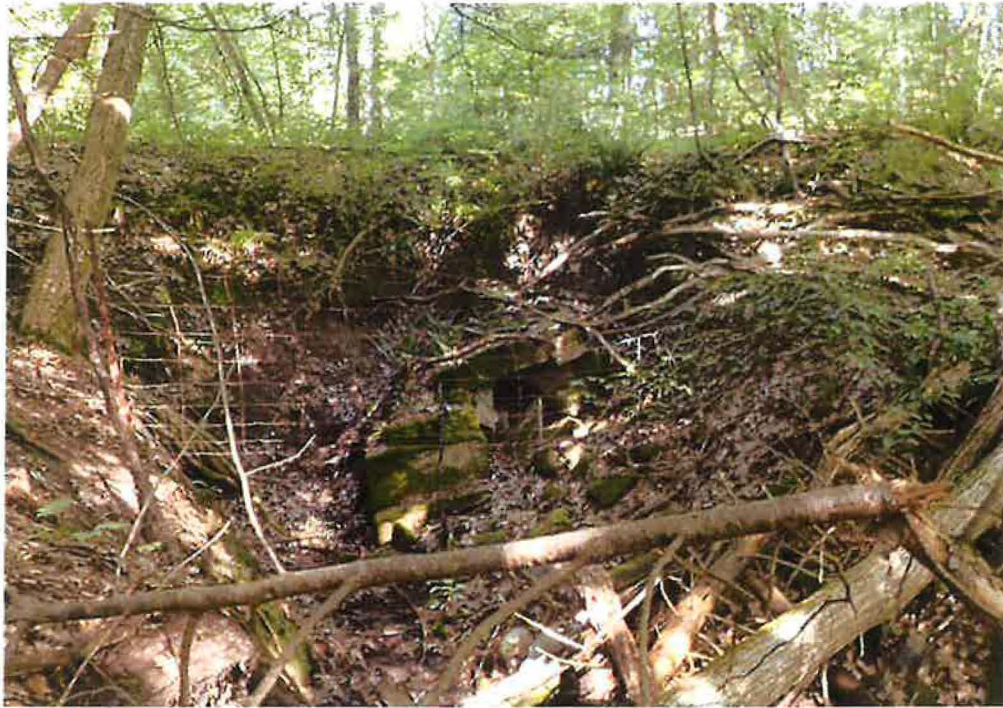
Photo 17: East Elevation showing Collapsed Section
