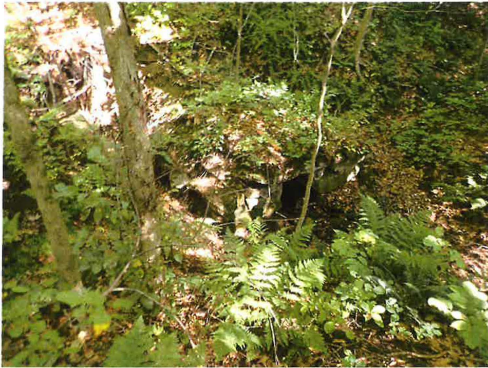
Photo 35: Erosion at East Side
