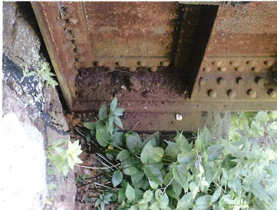
Photo 14: Tipped anchor bolt on the north abutment
