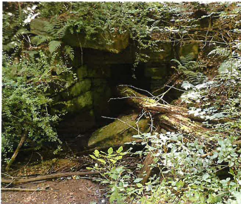
Photo 22: West Elevation Showing Southwest Wingwall Failure
