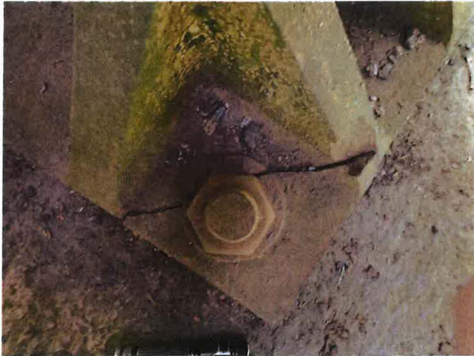
Photo 13: Cracked bearing on the bridge pier
