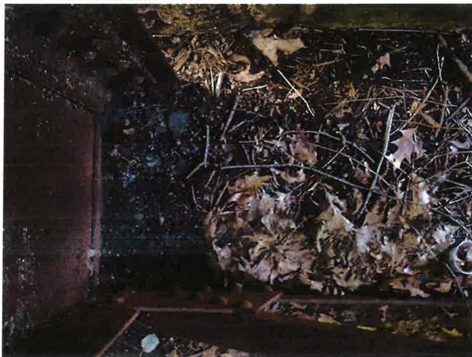
Photo 6: Heavy debris on bearing
