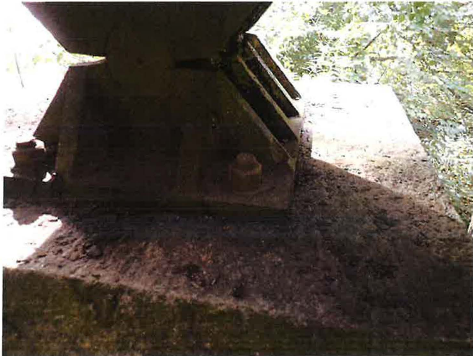
Photo 12: Cracked bearing on the bridge pier
