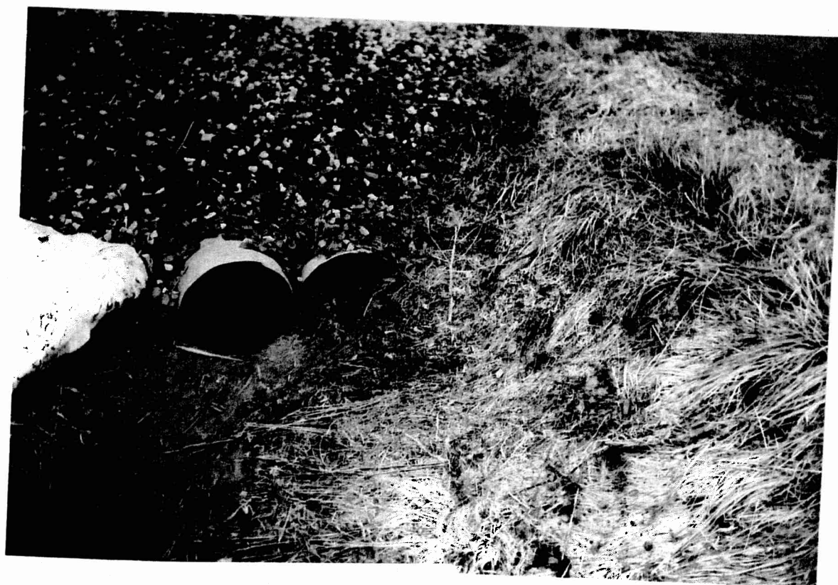
33. MP 394.1 Ontonagon River U823 – Double 34" Metal Pipe
