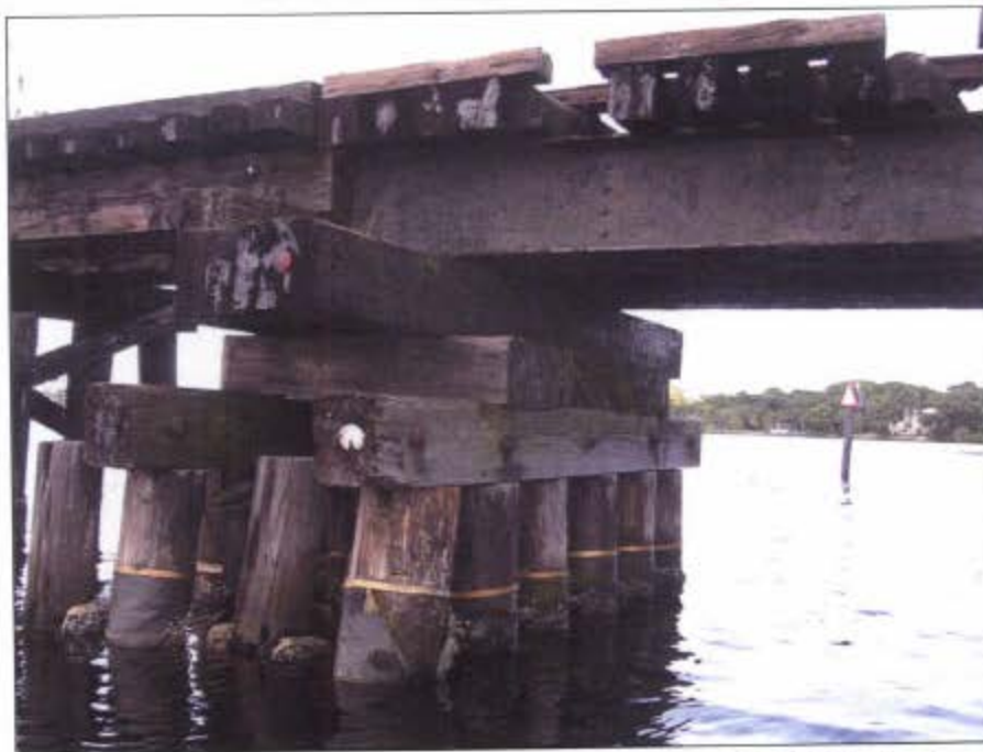
Figure 57. View of the timber trestle Railroad Bridge over Dona Bay (8SO5292), showing piles wrapped in rubber at low tide, oyster accumulation and rot due to ship worm, steel I-beam, reinforced bents with six piles, bolted caps and stringers, and missing ties at level of running rails, facing southwest.
