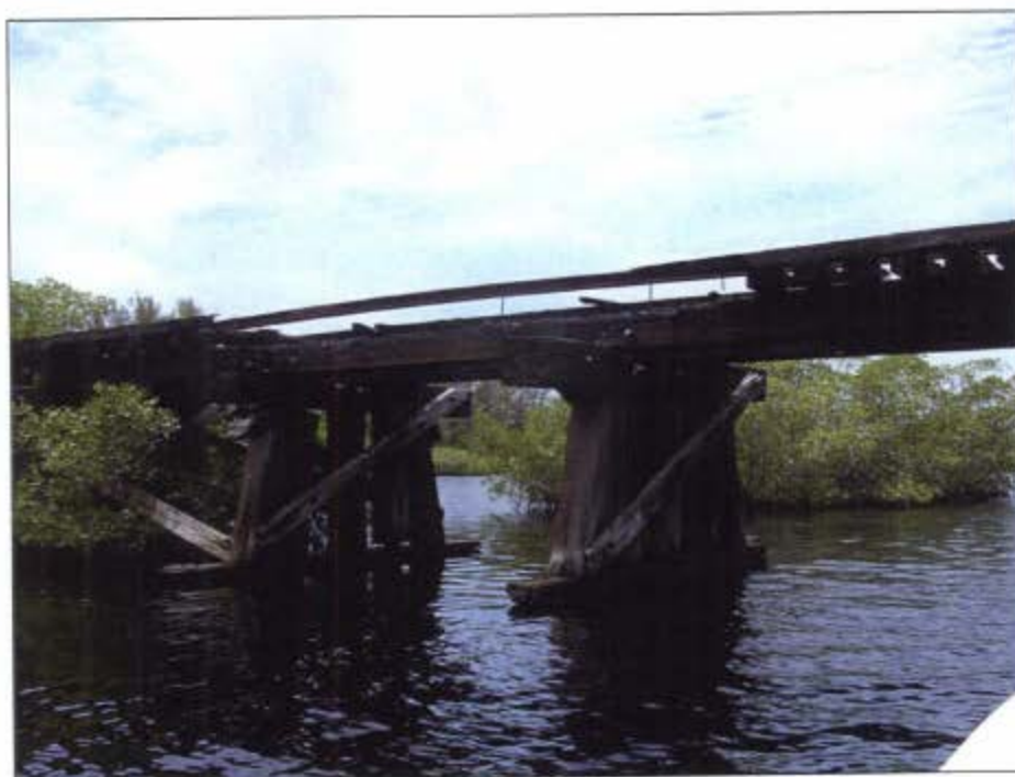
Figure 62. View of the Railroad Bridge over Roberts Bay (8SO5293), showing the burned portion of the bridge and square-hewn piles resting on stringers, facing south-southwest.
