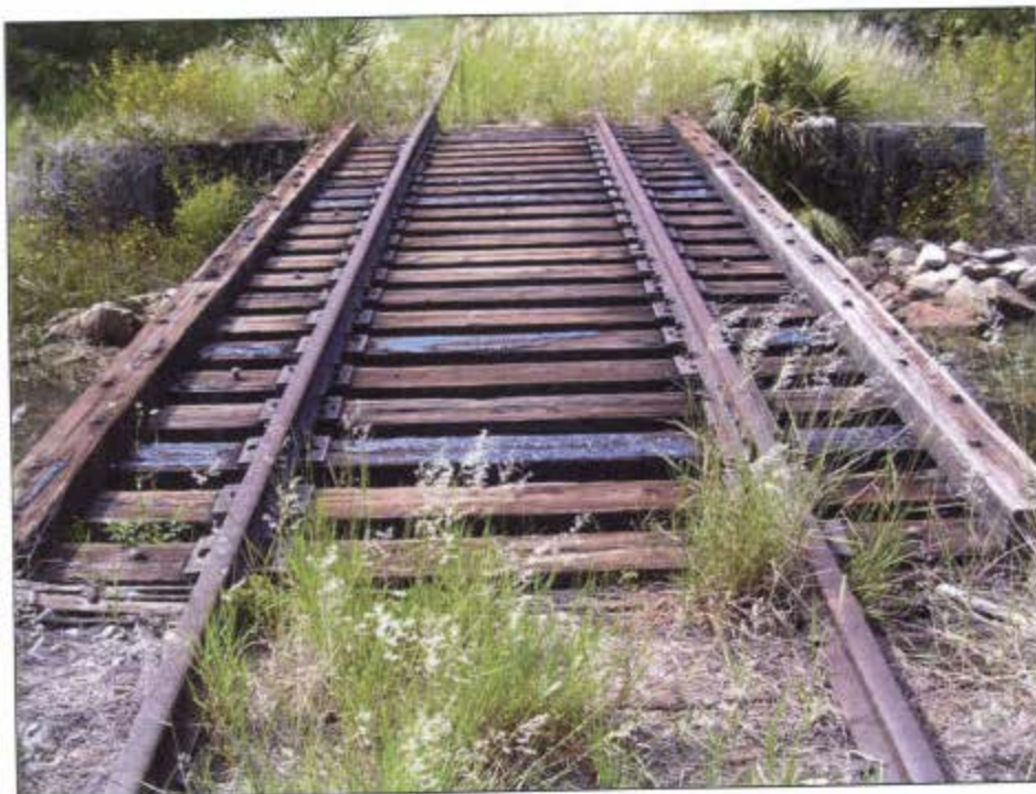
Figure 72. View of the short deck of 8SO5315, showing creosote or coal-tar brought to the surface of the ties by heat, facing south.
