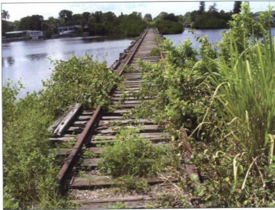
Figure 56. View of the deck of the timber trestle Railroad Bridge over Dona Bay (8SO5292), showing the deteriorated superstructure, facing south.
