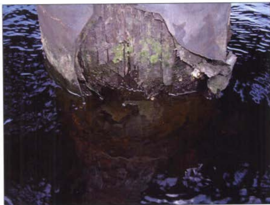
Figure 58. View of a rubber-wrapped pile, rotted by water and eaten by ship worms, Railroad Bridge over Dona Bay (8SO5292), facing west.
